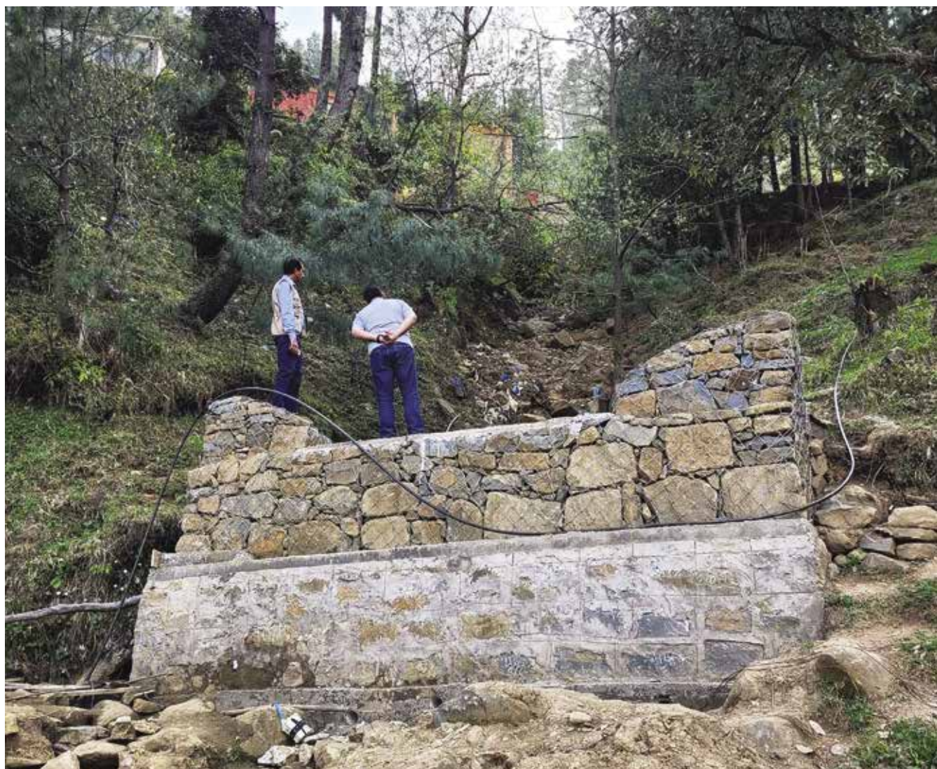
Islamic Relief worked with the local community to build this check dam above a village in AJK, where flash floods had previously destroyed four homes and a mosque. The dam stood firm in the 2022 monsoon, protecting 20–25 houses from harm
