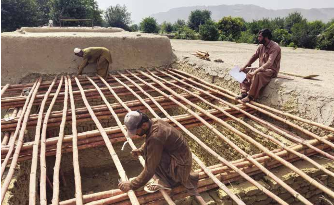
By July 2023 Islamic Relief had built 6,420 permanent flood-resilient homes in Balochistan and Sindh for families made homeless by the floods. Each includes a living space, kitchen and bathroom, and also features widened doors, a ramp and a commode chair to support the elderly and people with disabilities
